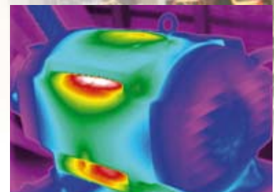
Abnormal uneven heating on motor
