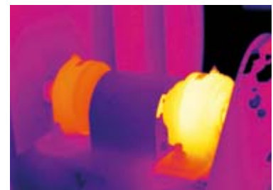
Overheating bearing cap
