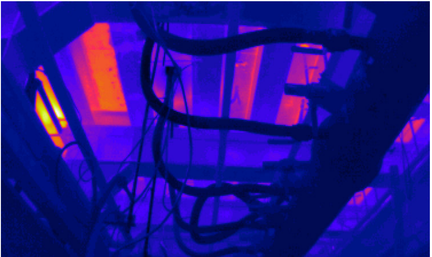
MONITORING OF TANK BOTTOM TEMPERATURES
