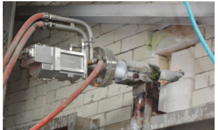
Fixed Installation of a process thermal imaging borescope
